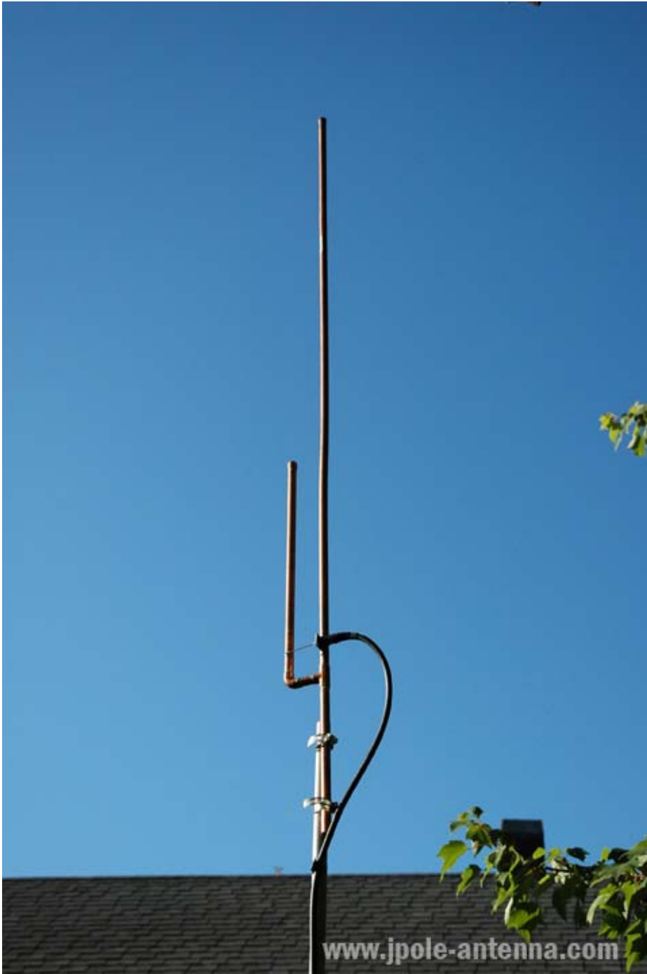
This J-Pole design is backwards. Notice the Shield is connected to the long element, and the center conductor goes to the shorter element.
